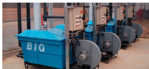
■ Low temperature boilers
